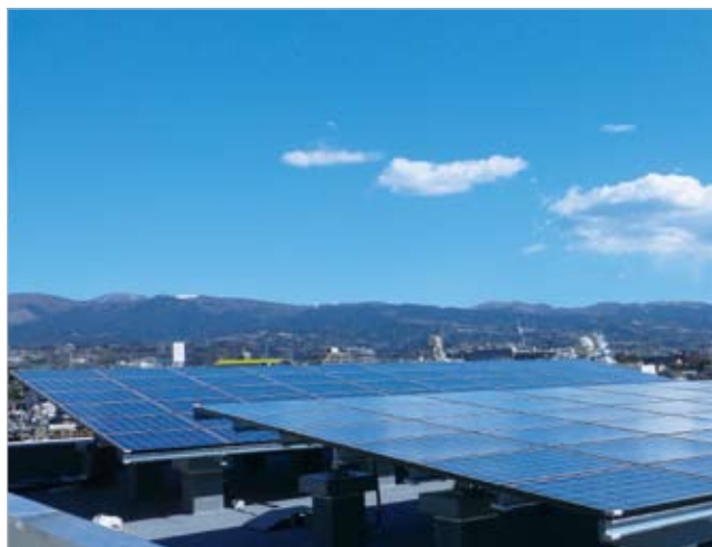
Solar power generation equipment installed at our Fuji Plant
