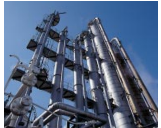
Distillation tower at the Yokkaichi Plant
