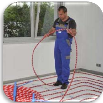
Radiant heating and cooling
