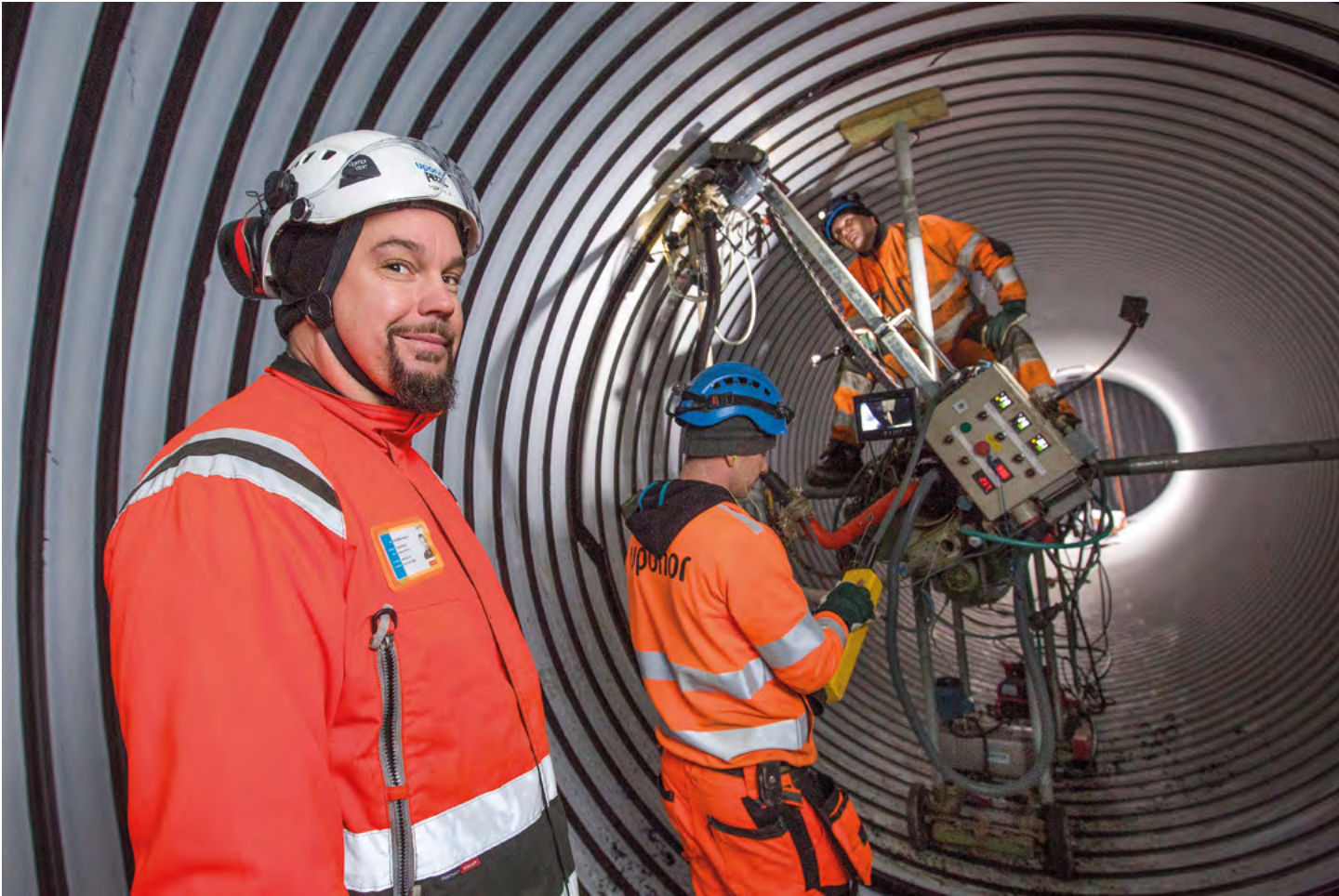
30m long Weholite® tanks were installed at a wastewater treatment plant in Riihimäki, Finland in late 2016. The tanks, each with an inner diameter of 3m and a volume of over 200m 3 , were installed to ensure that the plant can keep running even during emergencies.
