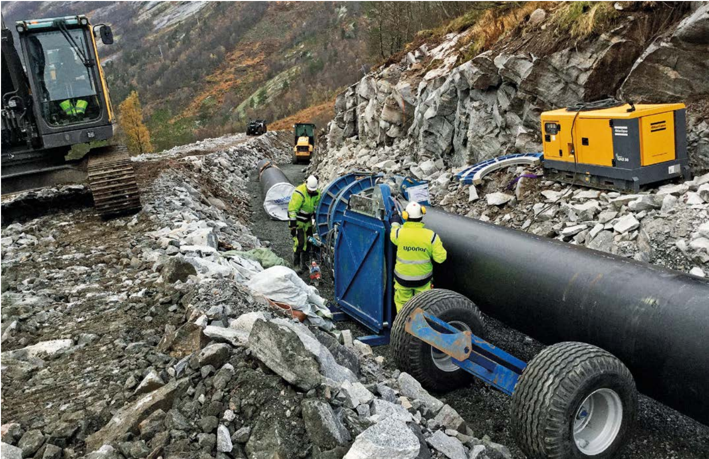
1.8km of Uponor's 1,000mm pressure pipe was installed in the demanding terrain of Glomfjord, Norway, to help the fertiliser producer Yara International renew water supply to its factory.
