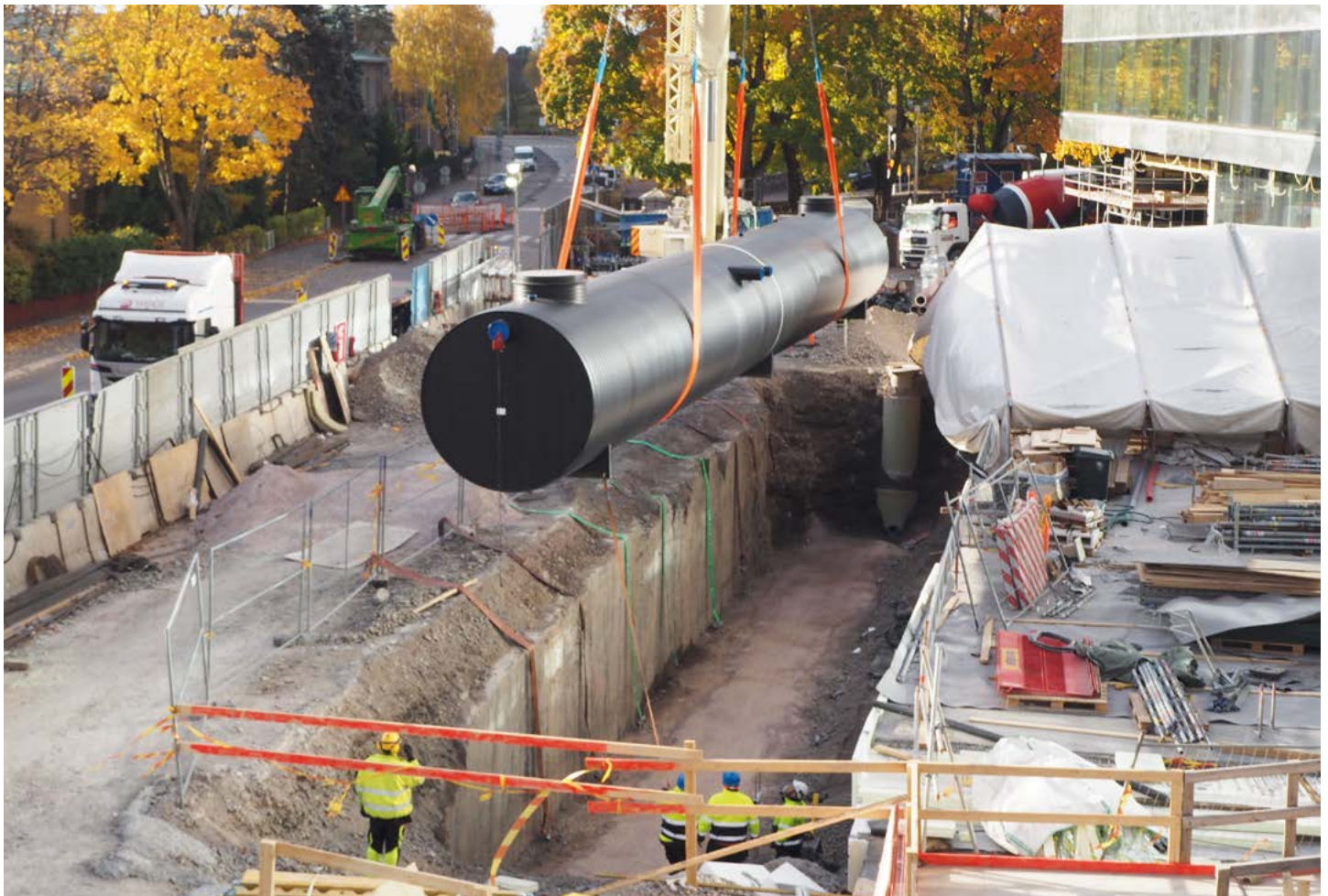
Uponor donated product systems to help build a new children's hospital in Helsinki, Finland. In October 2016, the hospital was equipped with a massive Uponor Weholite® storm water detention tank.
