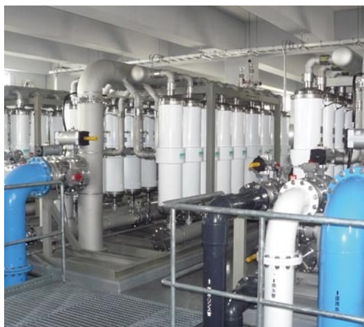
Kouzan Water Treatment Plant in Tottori, Japan
