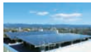
Solar power generation system installed at the Fuji Plant
