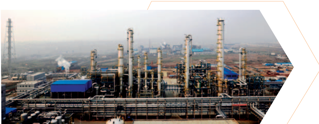
The above picture shows the 200 Ktpa syngas-to-glycol industrial demonstration plant of Sinopec Hubei Fertiliser
