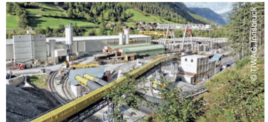
The run-of-the-river power plant on the Inn will make a significant contribution to Tyrol's energy autonomy.
