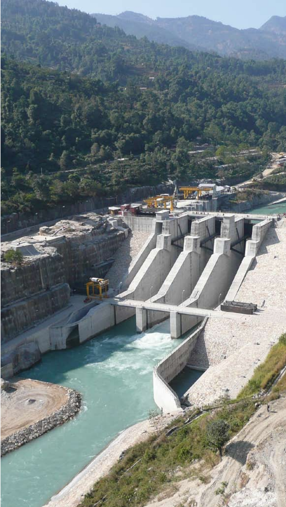
MIDDLE MARSYANGDI HYDROELECTRIC PROJECT, NEPAL
